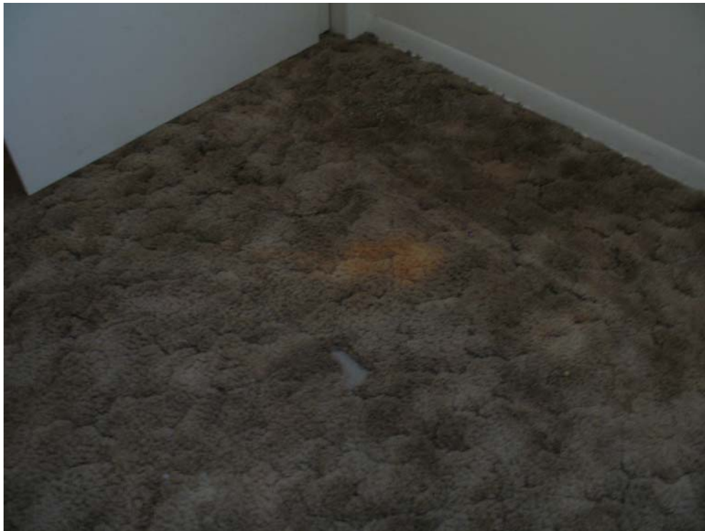
Photograph 1 Indicator Staining on Carpet
