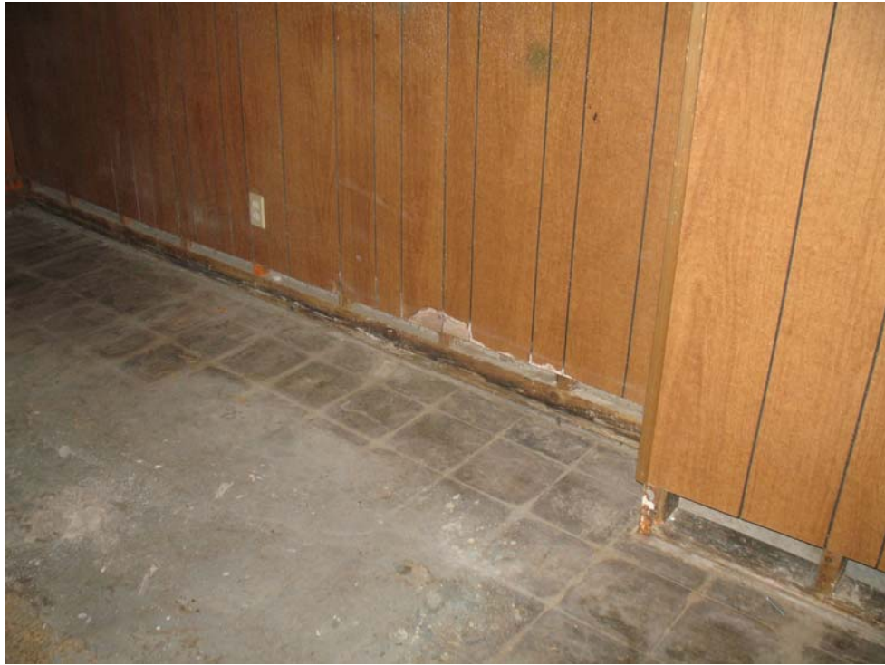
Photograph 3 Photograph of Basement Water Loss Indicators
