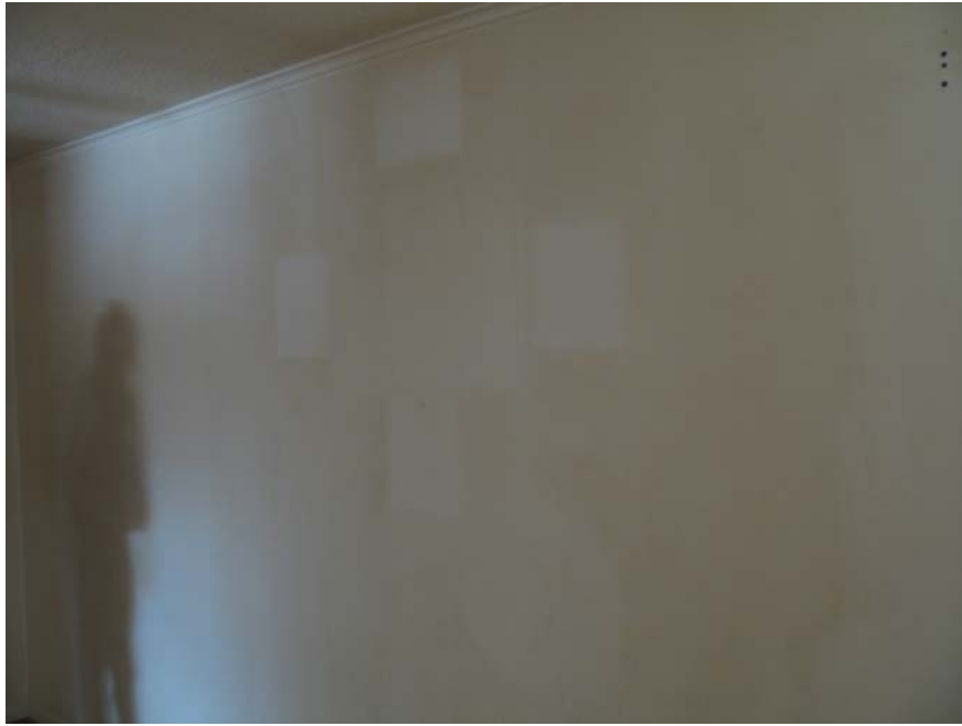
Photograph 2 Indicator Staining on Living Room Wall
