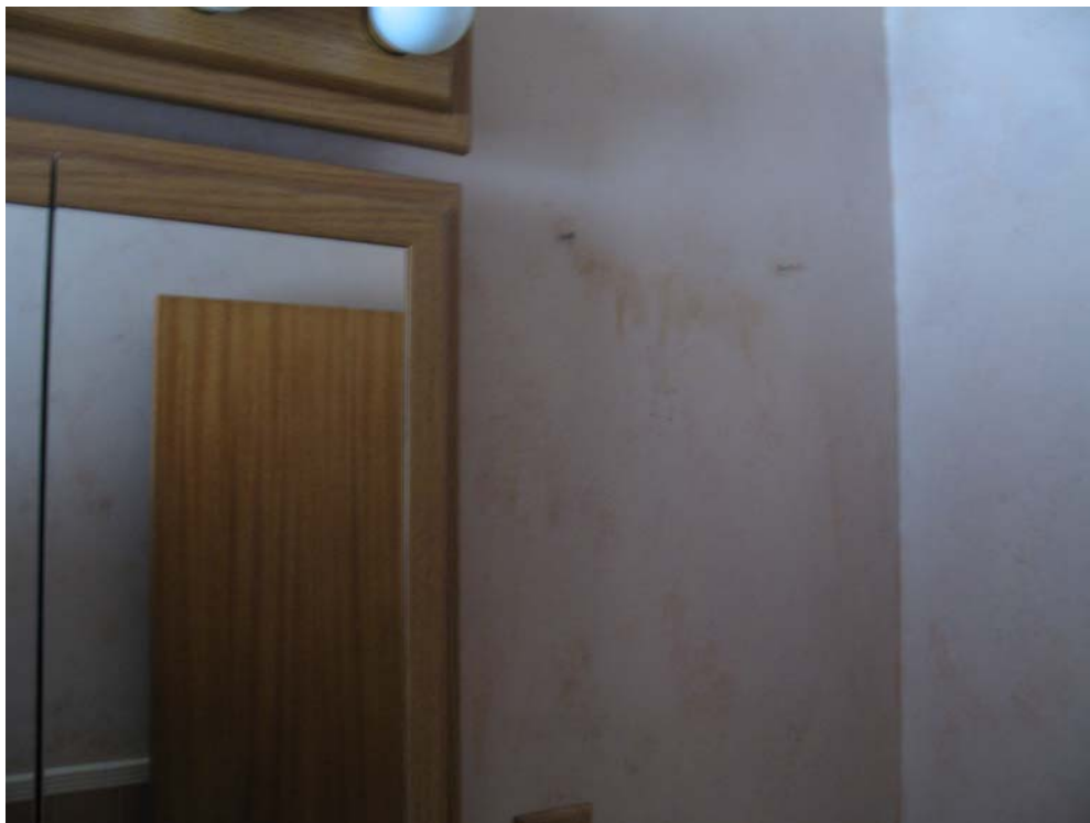
Photograph 2A Indicator Staining on Bedroom Wall
