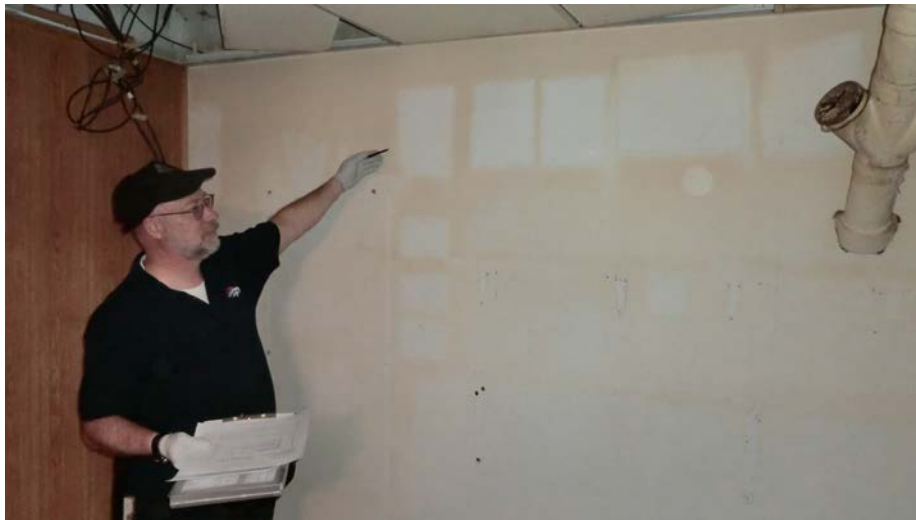
Iodine Staining Basement Living Room
