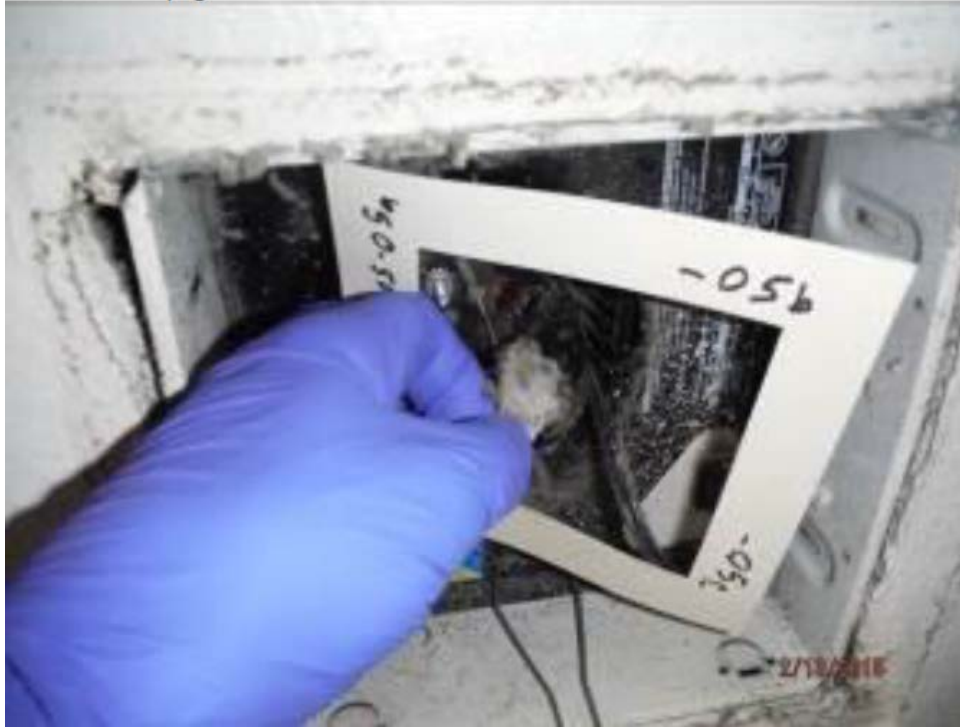
Photograph Documenting Failure to Collect 100cm 2
