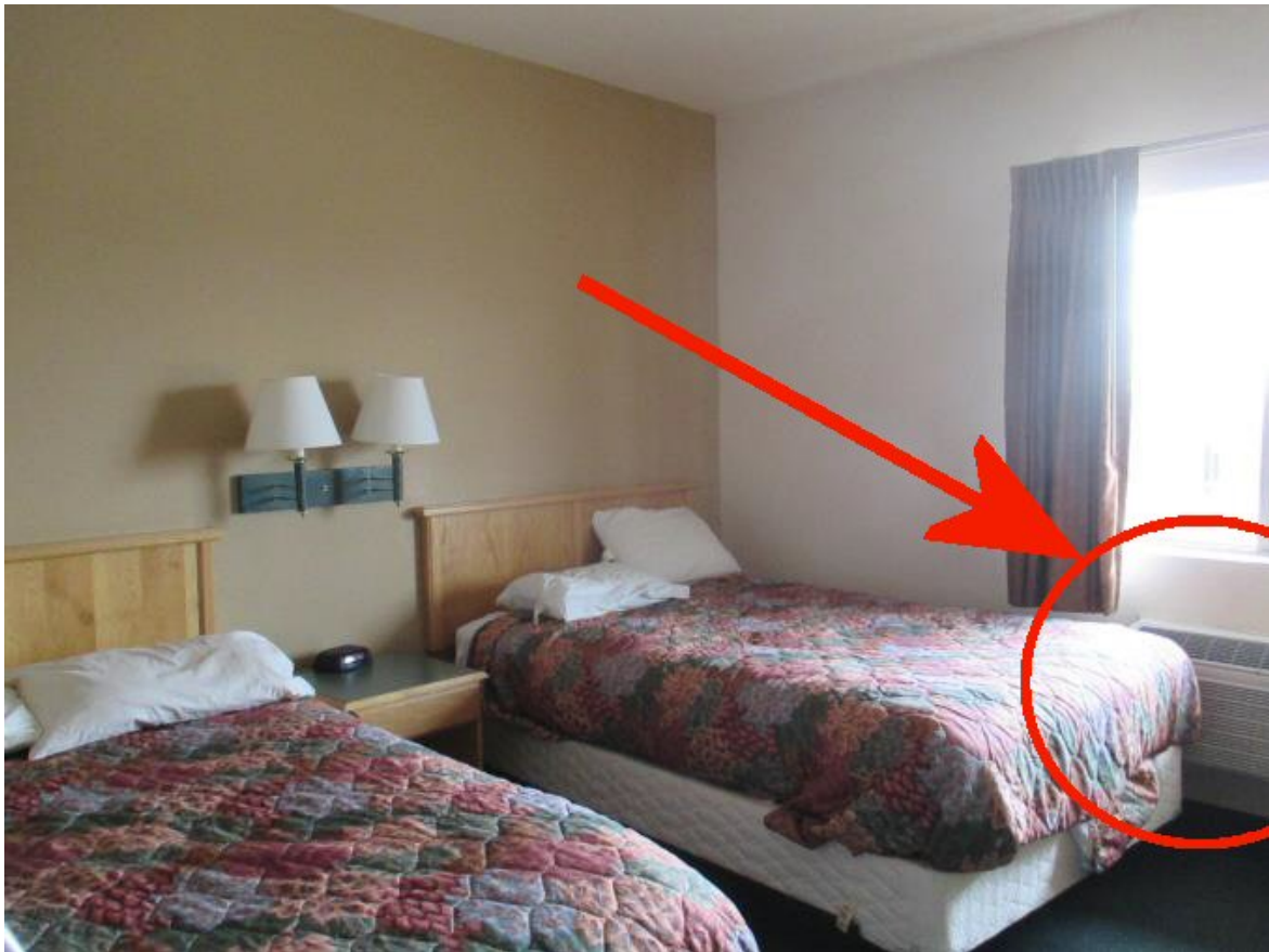
WEC Photograph of Non-ducted Heating or Cooling System
