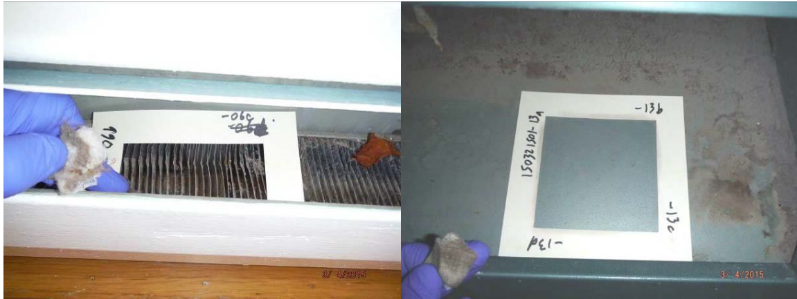
Quest Photographs Showing Remaining Dust After “Decontamination”
