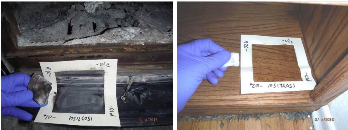
Quest Photographs Showing Remaining Dust After “Decontamination”
