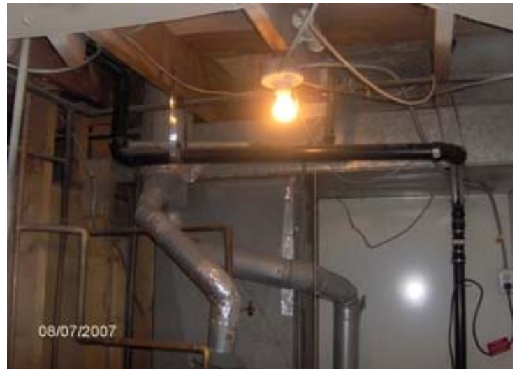
Area above furnace in laundry area
