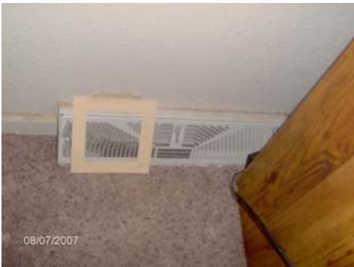
Supply duct along north wall east end of living room
