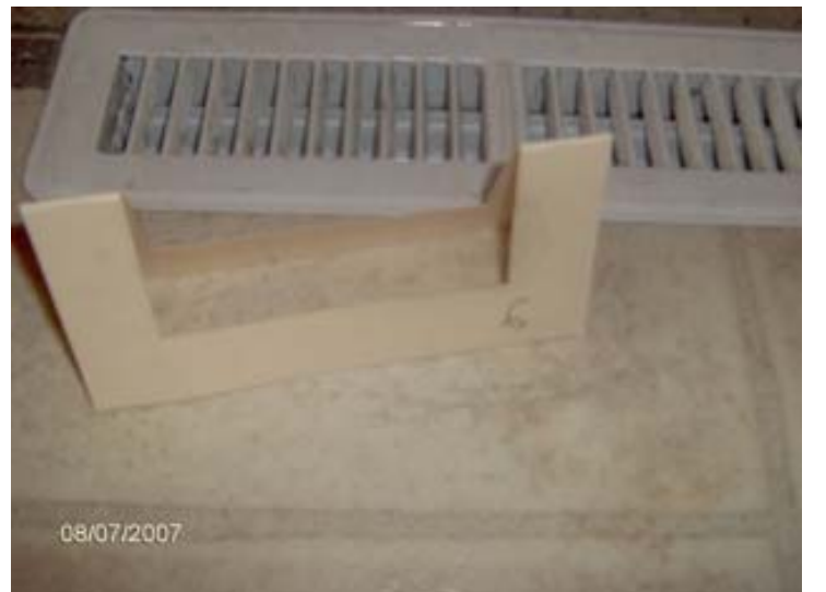
East supply duct between kitchen and addition
