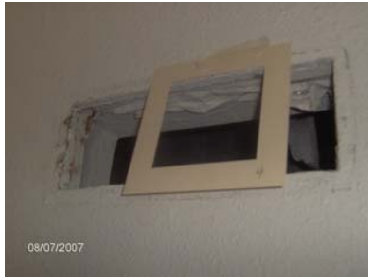
Supply plenum in living room along east end of south wall
