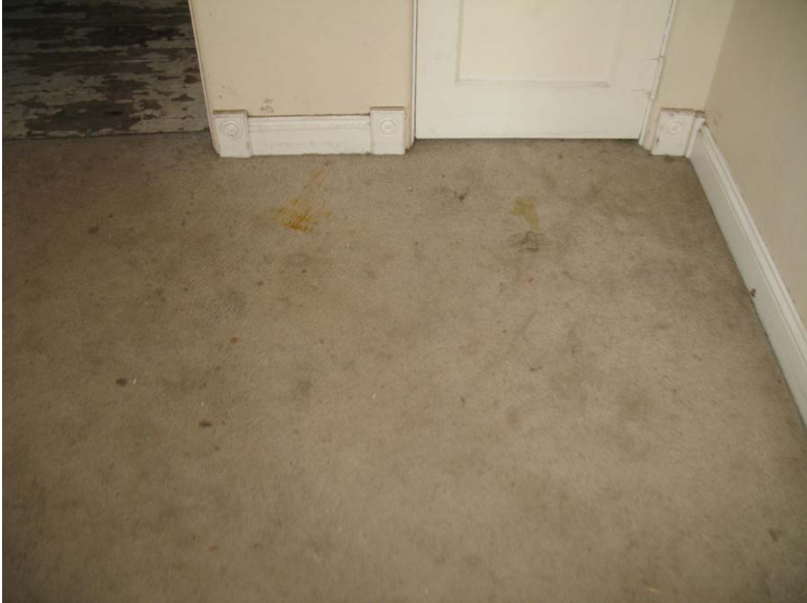
Photograph of Iodine Staining at 1170 Garrison Street Lakewood, Colorado 80215 18
